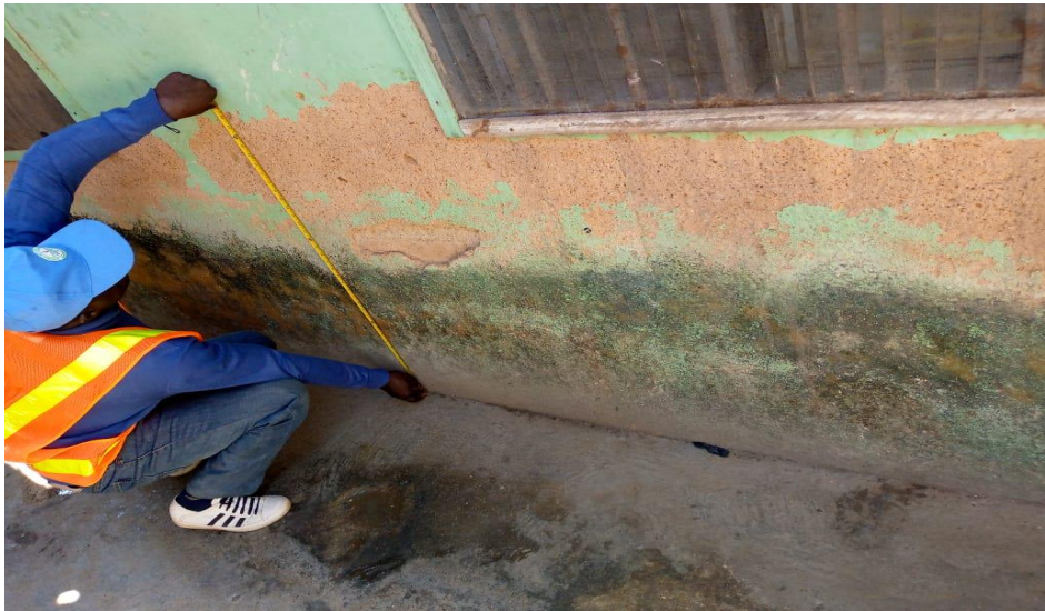
Plate 3.0 Staff measuring the height of dampness and presence of mould growth
