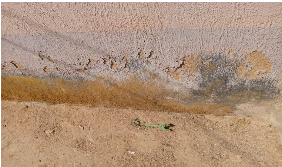
Plate 2.0 Presence of efflorescence on the wall and peeling of mortar
