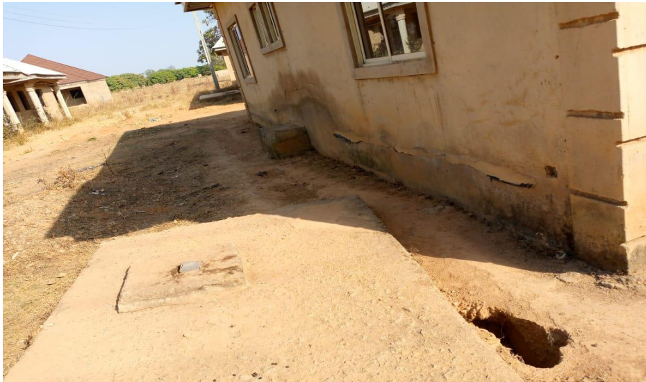
Plate 1.0 Presence of dampness at the base of the building
